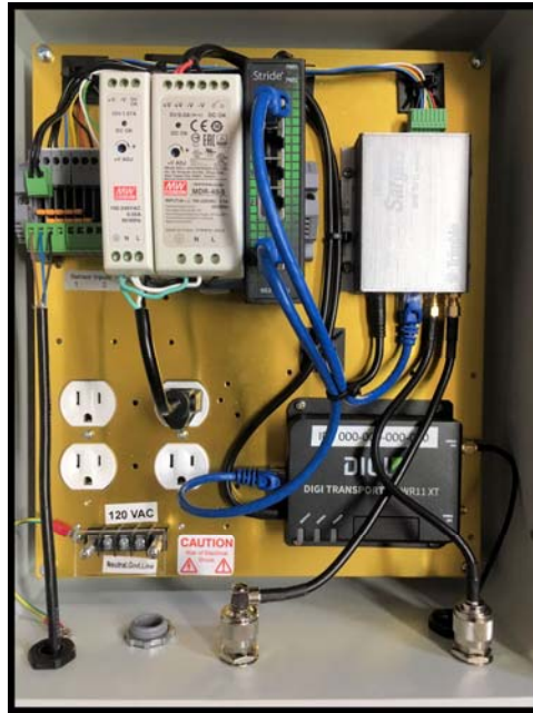
Figure 2 - Inside the Weatherproof Enclosure
